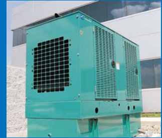
Back-up Generator Power
