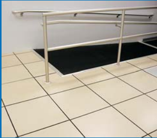
Raised Floor Environment
