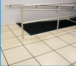
Raised Floor Environment
