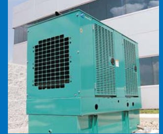
Back-up Generator Power
